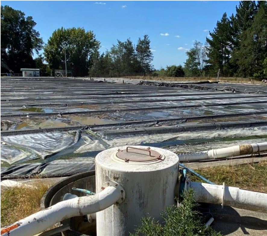
Figure 5: Fonterra's Tirau Anaerobic Lagoon Digestion Plant
